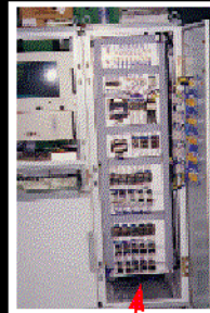
Load center for pump/heater control
